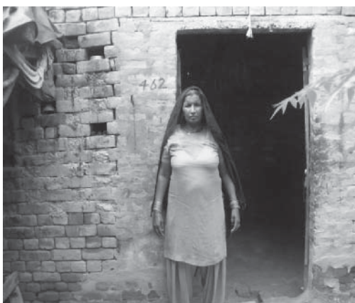
Poorly finished structure
