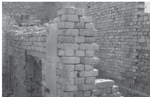
Poor quality building material
