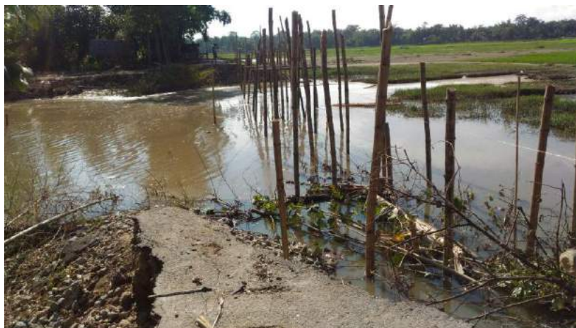
Broken pucca road passing through Kohuadoloni cutting off road connectivity to many villages
