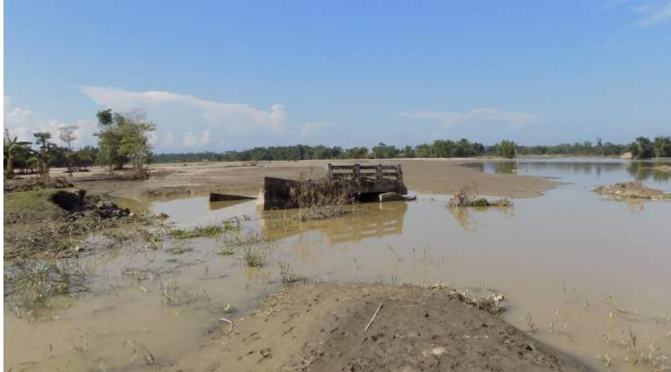
A broken culvert
