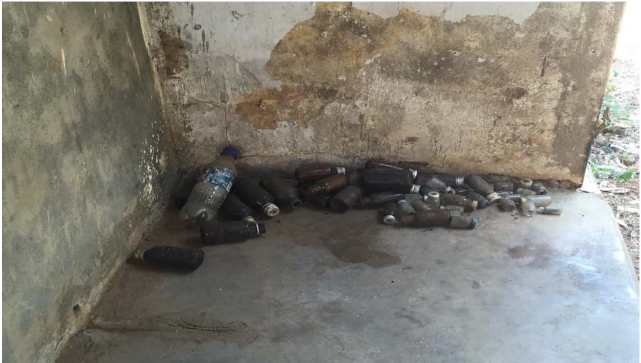
Improper disposal of old medicine bottles in a corner of the CHC immediately next to the labor room and operation theatre.
