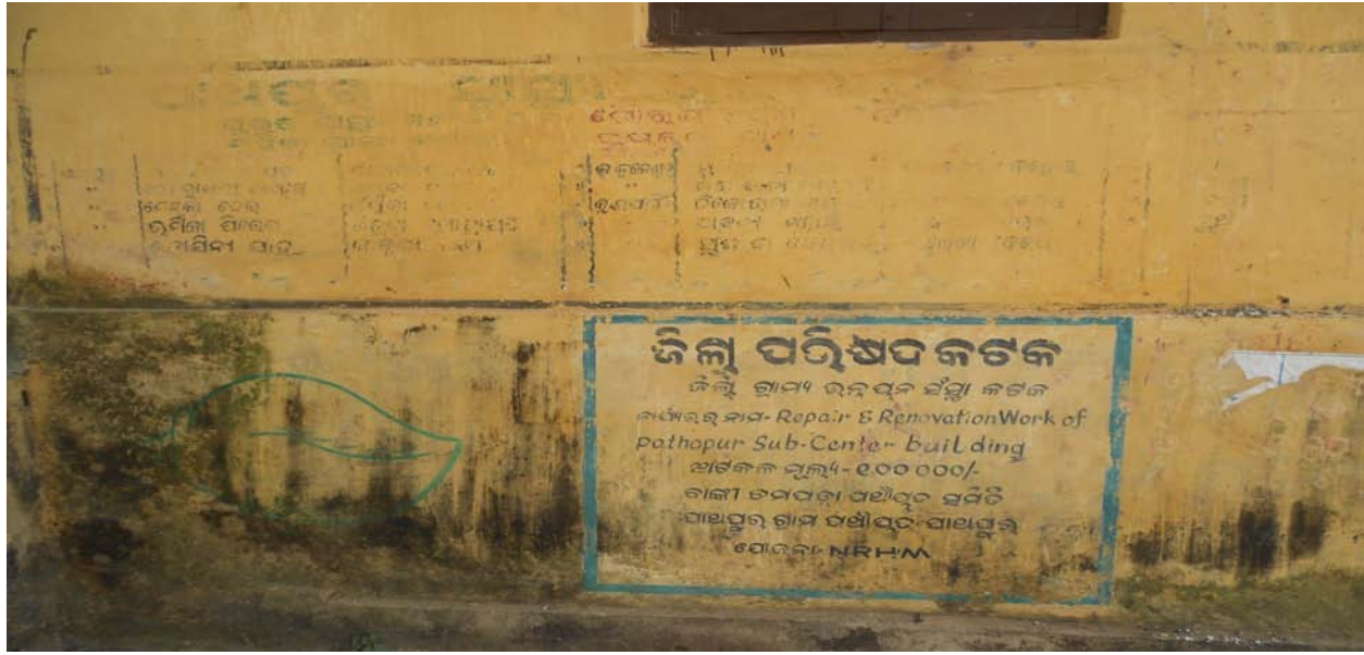
The signage is worn away because no one maintains the building.
