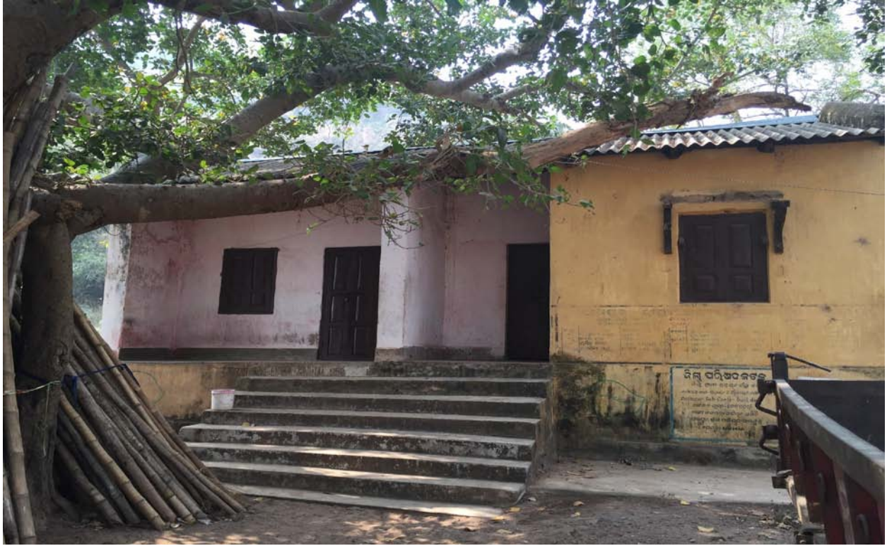
The Pathapur sub centre is closed and in a state of disrepair.
