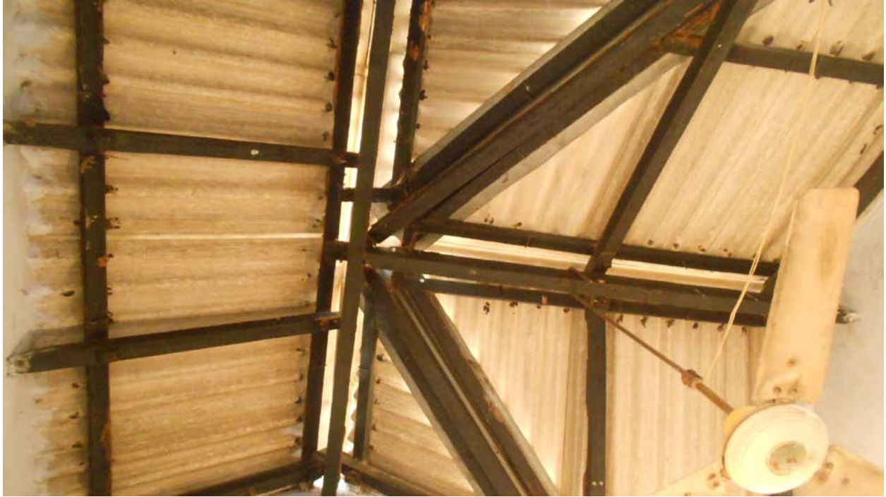
Ceiling in the Immunization Room with gaps where rainwater, fecal matter from birds and monkeys, and other debris enter the room, exposing medical staff, patients and the medicine to harmful environmental elements.
