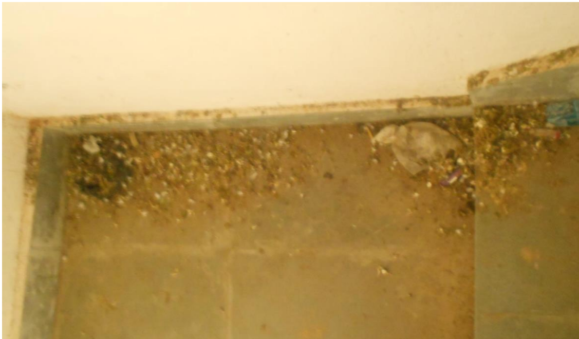
Debris and animal/bird fecal matter in the stairwell leading to the AWC
