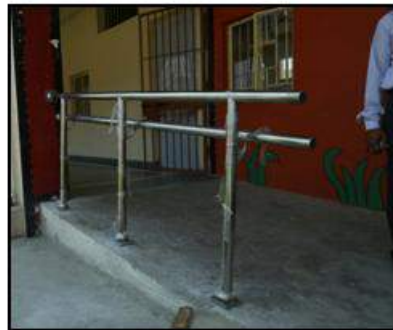
Presence of a ramp of an appropriate slope with hand rail on one side at two levels leading to Ward No. 1 (Mandoli Jail)
