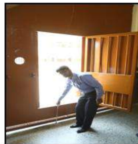
In accessible entry via the small iron gates. Small iron gates at a height of 17" from the floor surface. (Rohini Jail)
