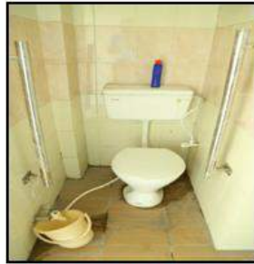
Accessible washrooms with grab bars at both sides at a distance of 24"; accessible wash basin and doorway (Mandoli Jail)
