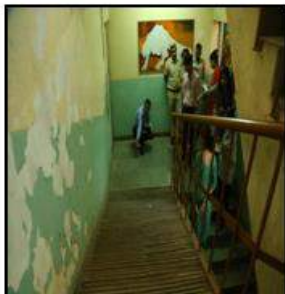
Presence of the Meeting room on the second floor, completely inaccessible to wheelchair users. And an unsystematic and unexpected presence of a steep ramp in between flight of steps connecting two floors. (Rohini Jail)
