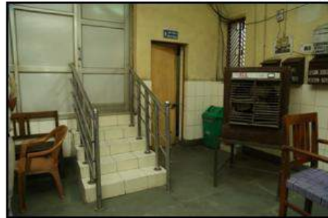
Air cooler obstructing the passage to the washroom Distance of only 22" between the cooler and handrail. Flight of five steps leading to the Shinakt Kaqsh with abruptly ending handrails (Rohini Jail)
