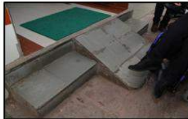
Entrance to the medical facility has a steep ramp (Tihar Jail)
