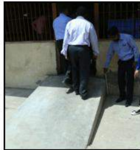
Presence of a ramp at a height of 13" towards the Canteen and the Press Room (Mandoli Jail)
