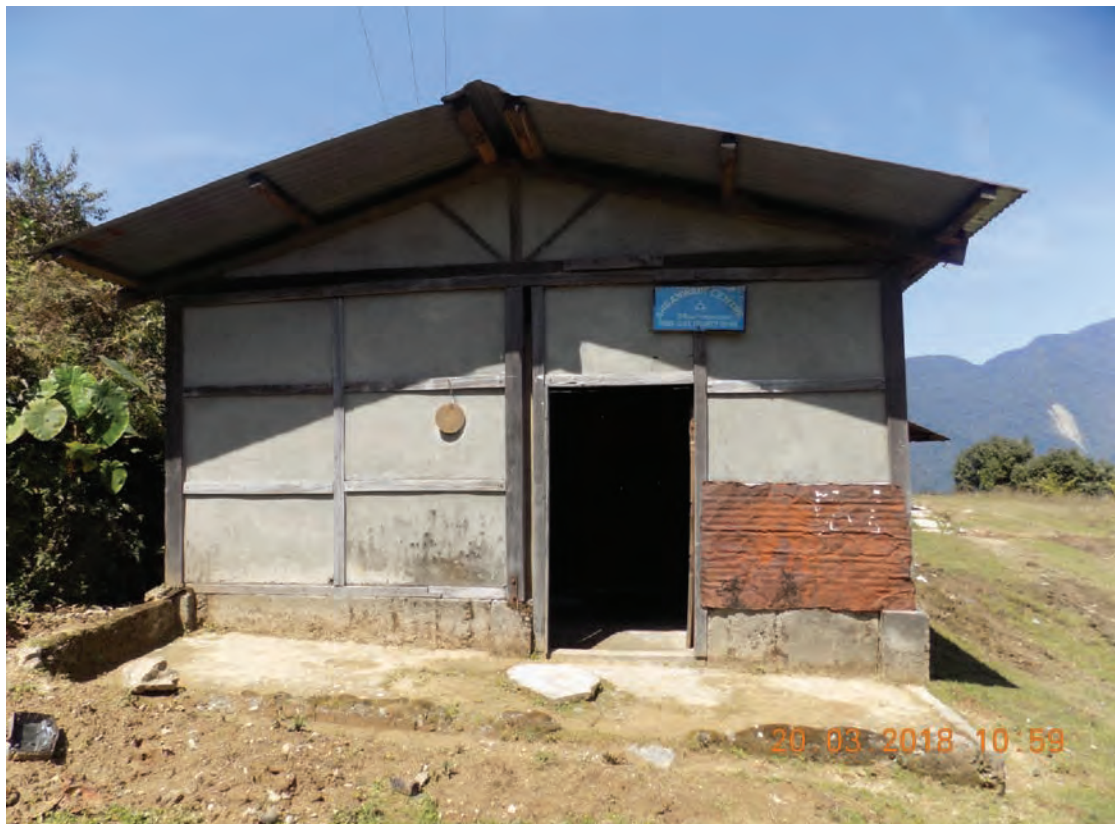
Non functional Anganwadi Centre, Tiwari Gaon, Arunachal Pradesh
